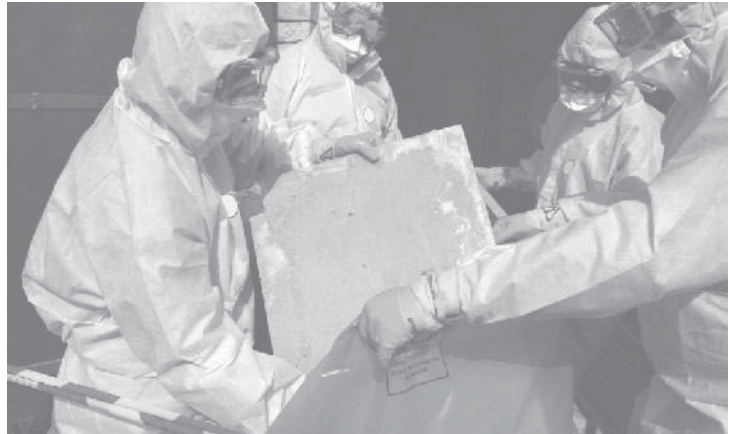
The Asbestos Management Toolkit assists non-profit housing providers in creating their own asbestos management program.
