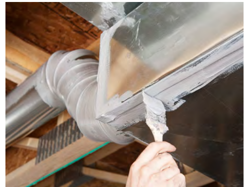
Figure 9: Duct sealing: It is important to seal all seams and joints with a durable aluminum foil tape or a liquid sealer or mastic, to ensure that the ductwork supplies and exhausts the quantities of air per the design.
