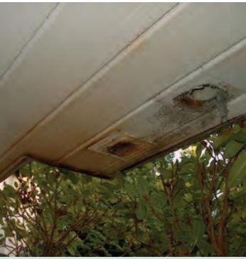
The build-up of debris or dirt on the underside of the balcony limited the air flow through the vent, resulting in damage.
