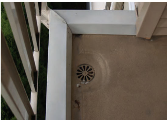
Maintain drains free of obstructions, dirt or debris to ensure they are free flowing and to prevent water ponding.
