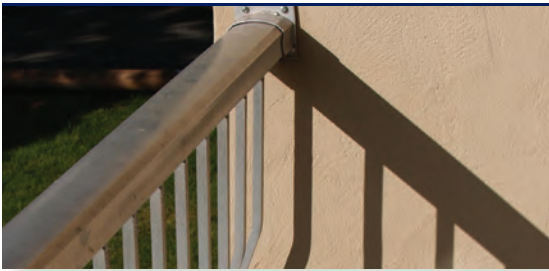
Guardrail connection to the wall can be a vulnerable point of water ingress.
