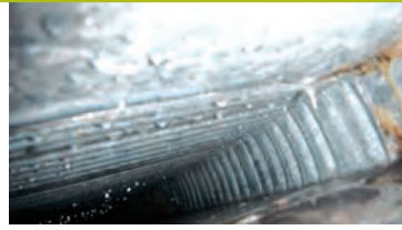
Condensation at the duct outlet.
