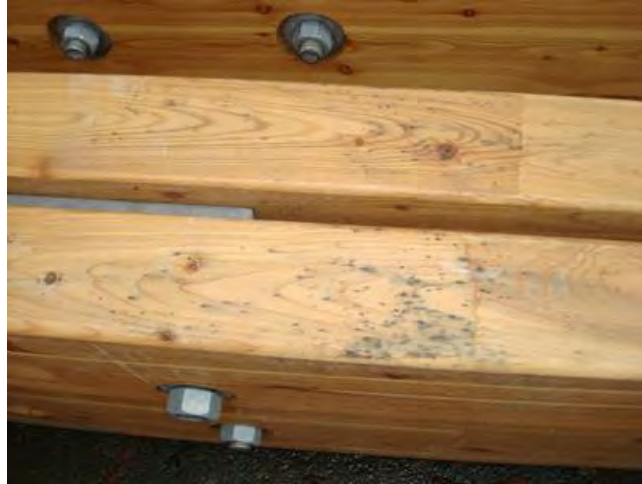
Figure 5 Iron staining on glulam
