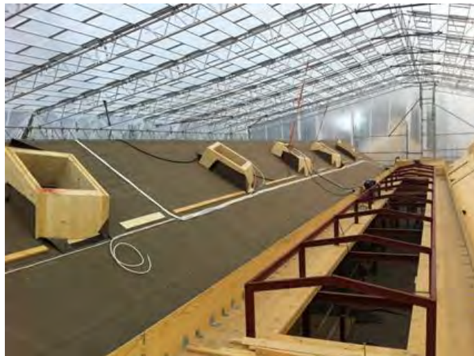
Figure 12 Using a fixed temporary roof to protect roof construction in Norway (Photo courtesy of Fristad Bygg)
