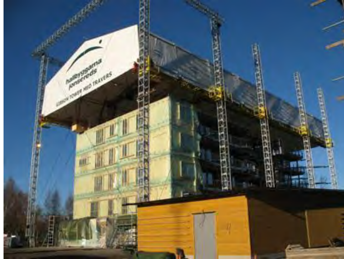
Figure 13 Using a movable temporary roof to protect the entire construction in Sweden
