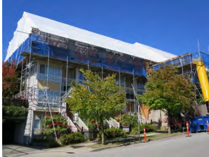
Figure 11 Weather protection using a fixed temporary roof during retrofit of a building in Vancouver
