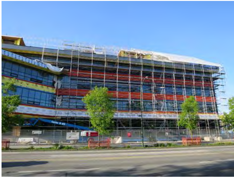
Figure 10 Using a tent to protect roof construction in a recent Vancouver project
