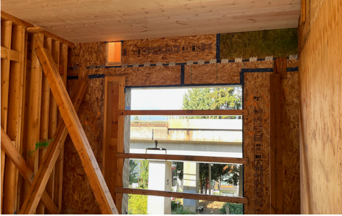
Figure 6. Interior of a suite with wall panel for above level attached. (source: Scius)
