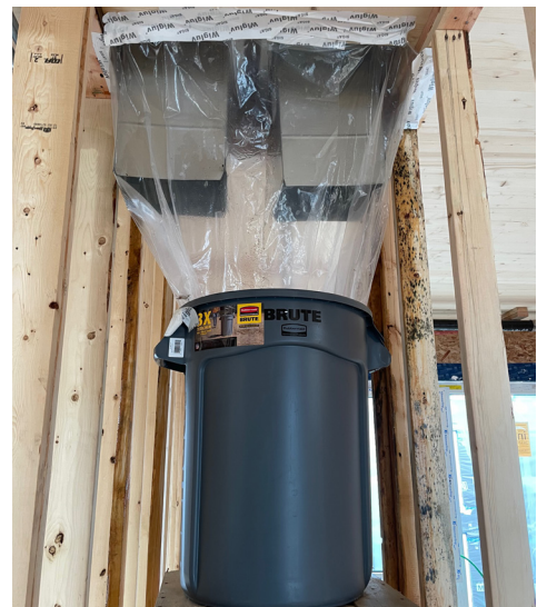
Figure 19. Collection of water seeping in from ducts (source: Scius)
