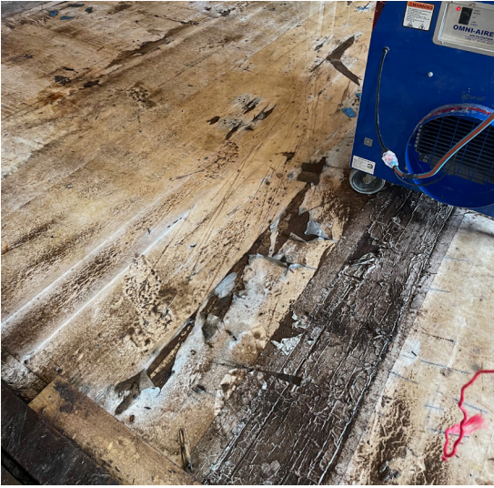
Figure 17. Damage to weather protection membrane on the CLT (source: Scius)
