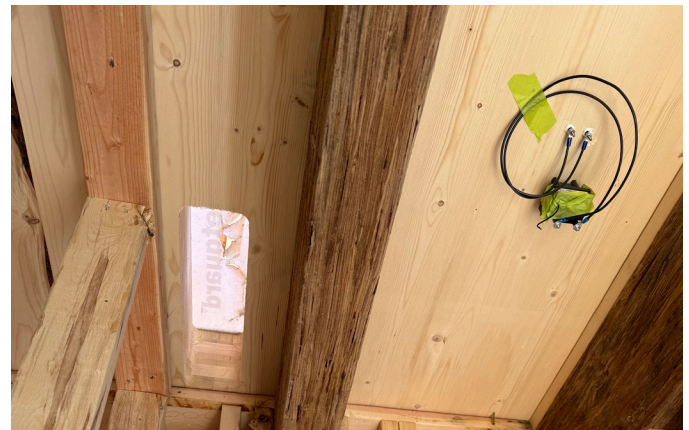
Figure 15. Sensor installed on CLT in electrical closet (source: FPIInnovations)
