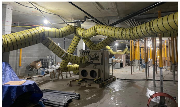
Figure 20. Dehumidification system installed in the parkade (source: Scius)
