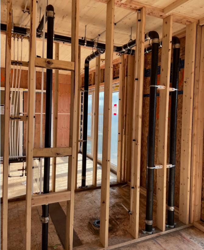
Figure 6. Plumbing in a Vienna House washroom. (photo: Scius)
