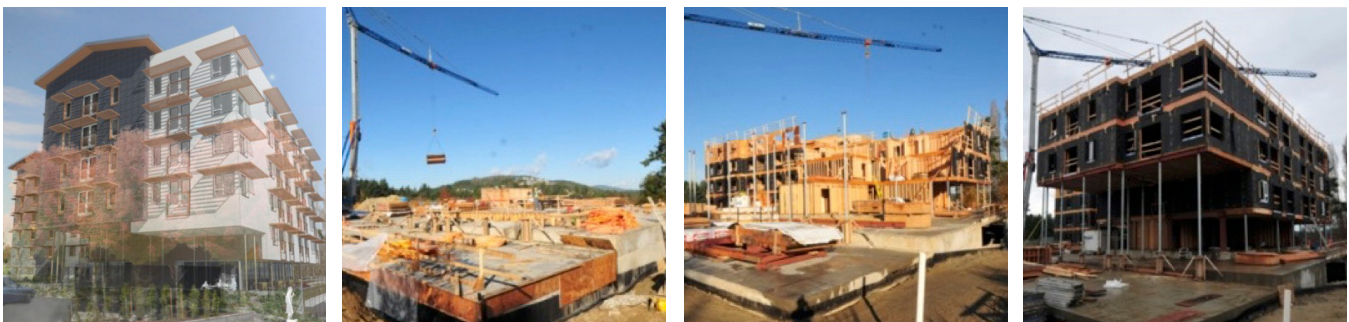
Image sequence, left to right: rendering to construction progression, Southeast elevation. (Rendering source: Cascadia Architects, progression photo source: Multivista)
