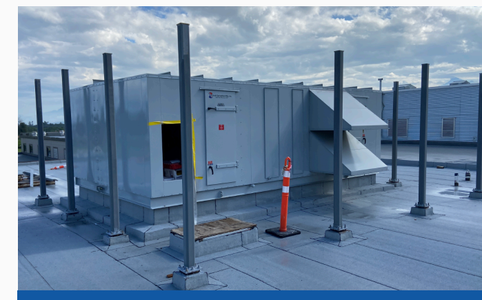
Figure 7. Figure showing anchor penetrations into the roof.
