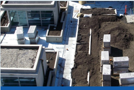
Figure 3. Accessible Rooftop Photo of exposed concrete parapets and concrete planter walls that bypass the thermal insulation.
