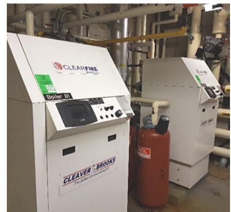
Two Hydronic Boilers in MURB Building
